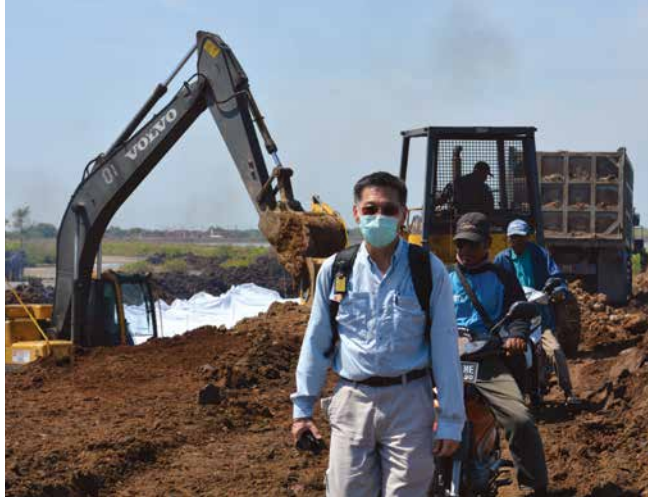
Prof Karl Kim and team observe the continuous levee construction. Photo credit: Rita Padawangi
